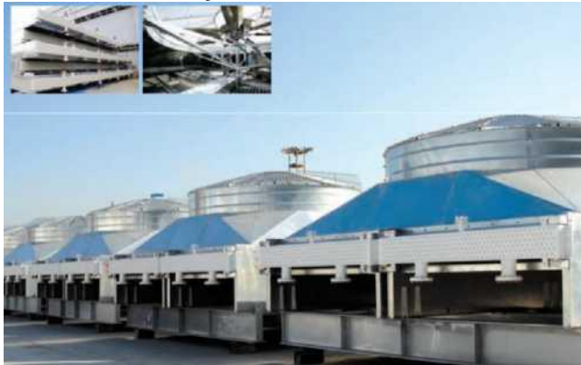
Air Cooled Heat Exchanger
